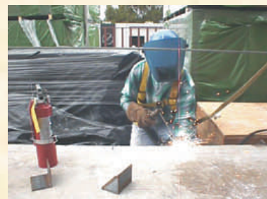
Proper Personal Protective Equipment should be used when welding. Notice this worker is wearing a welding shield, leathers and he has a fire extinguisher nearby his hot work.
